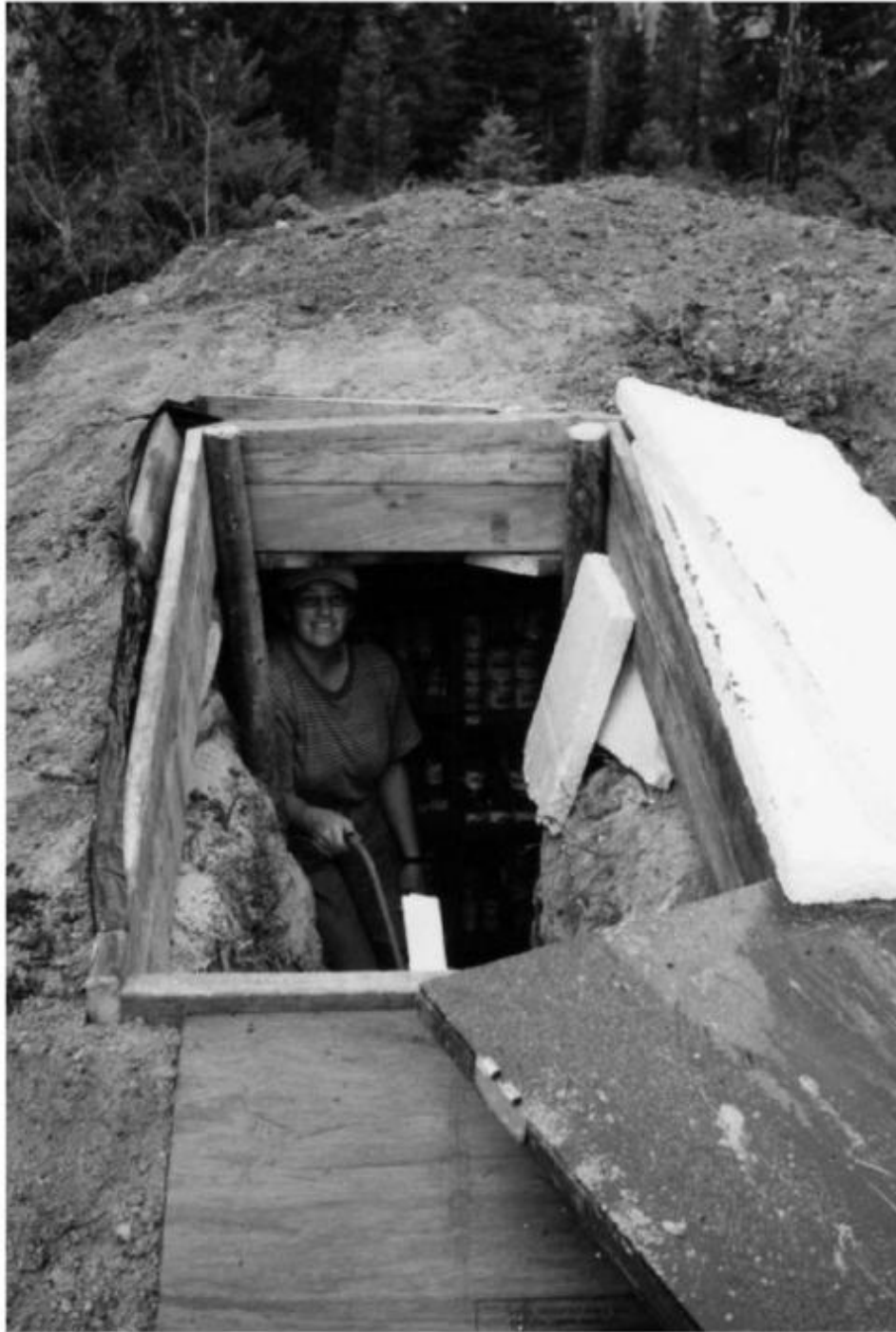
Our hand-dug root cellar is perfect for keeping things from freezing. This photo was taken during our first winter on the homestead, so the food inside was store-bought rather than home canned or produced.
